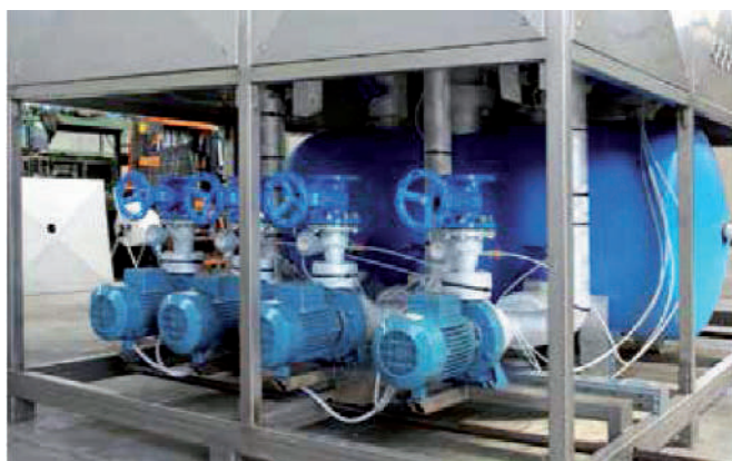
Raca Plus Energy chiller pumping units
