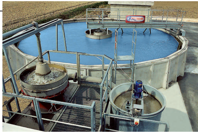
Water treatment/recycling system with 60-70 m³/h capacity, ancillary to polypropylene big-bags and LDPE film recycling line 1000-1200 kg/h
